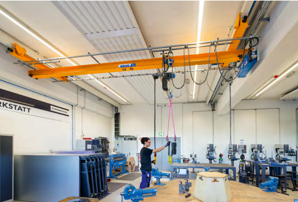
Underslung travelling crane with electric chain hoist, a sturdy rolled section girder and main girder connection version 1
