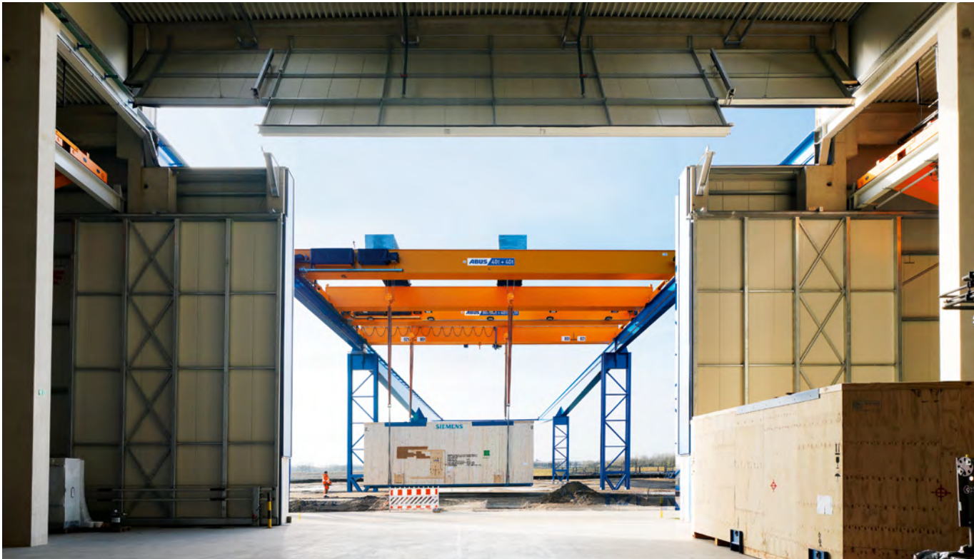
When travelling outdoors, a control circuit operated via the ABUS overhead crane controls the crane flap interlock system
