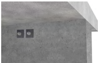
View of rear of standard bracket fitted to reinforced concrete support
