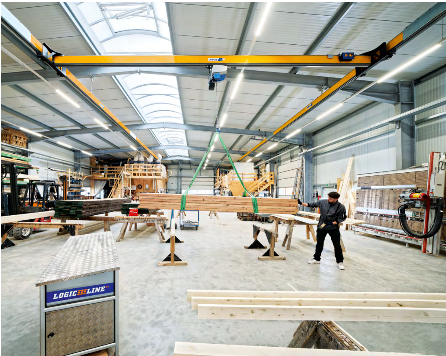
Fitted to rolled section I-beam using clamps
